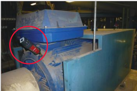
Lubrication of pump motor
